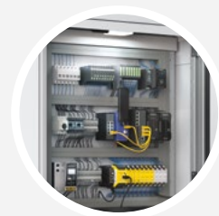
Control panel technology, DIN rail terminal blocks
